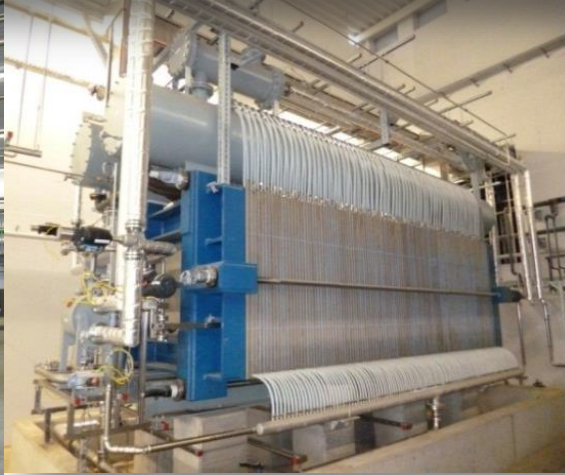
One of three 2MW el electrolyzers
