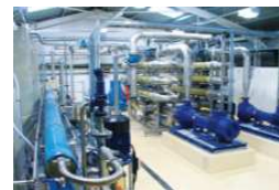
Water filtration systems
