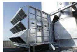
Air filtration systems
